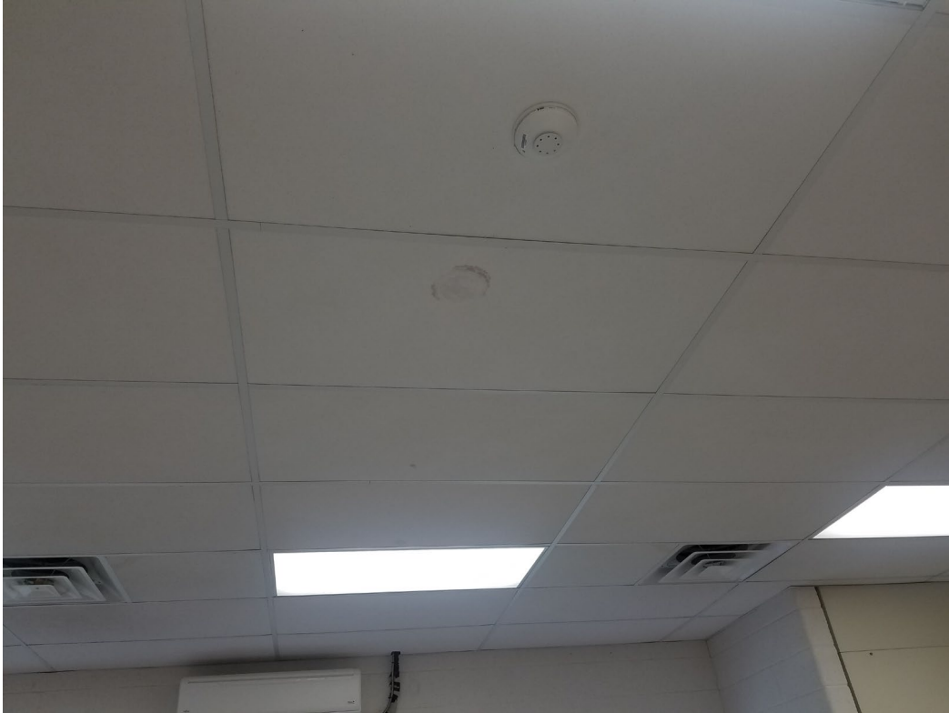
#1 – Staining on acoustical ceiling tiles (typical conditions).
