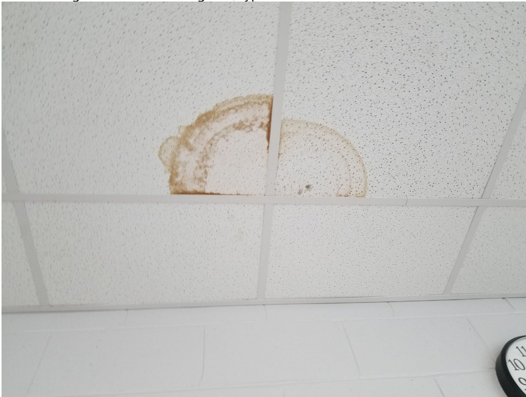
#2 – Staining on acoustical ceiling tiles, typical conditions.
